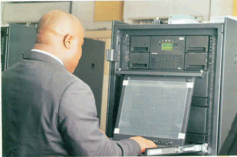
Server Room, CSCS Head Office
